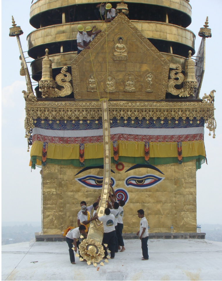
Fig. 3. The western side of the harmika of the Swayambhu chaitya, Kathmandu, Nepal, on conclusion of the renovation in June 2010 showing workers hoisting an honorific banner, executed in gilded brass, in the name of Tarthang Tulku, Head Lama of the Tibetan Nyingma Meditation Center at Berkeley, which sponsored and oversaw the chaitya's renovation from 2008 to 2010; photograph provided by California Nyingma Institute
